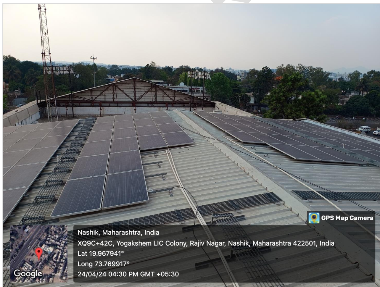
Plate 5: Rooftop solar panels in the premises
